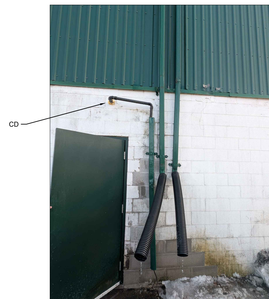
REFERENCE IMAGE - EXISTING EXTERIOR CONDENSATE DRAIN
